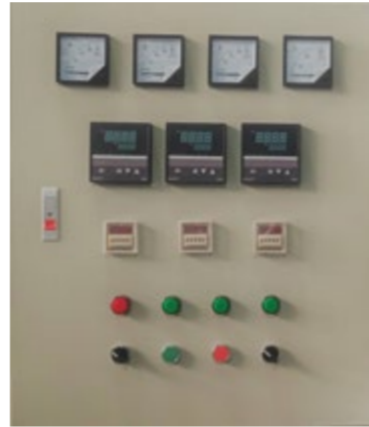
传统电箱 General electric box
